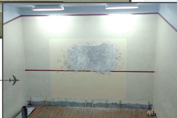
✈ Bad condition plaster court, before renovation
